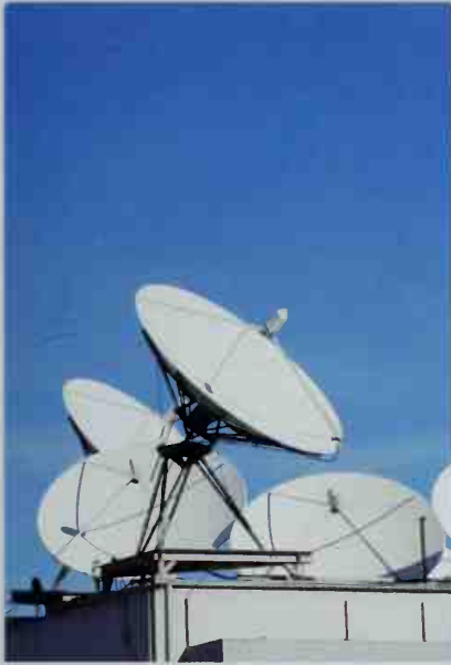
■ A parabolic radio antenna: This sort of transmitter creates a highly focused and strong signal.
