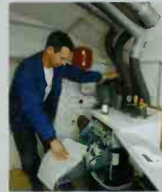
■ A heat pump in a single-family home, with control module, hot water, and buffer storage systems.
