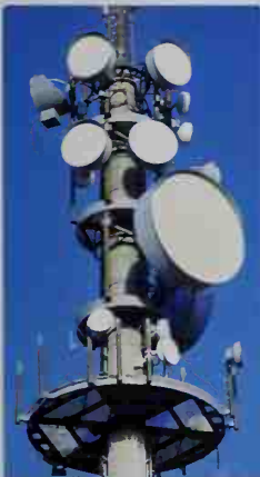
■ Crowded transmission masts can often be seen in urban areas.
