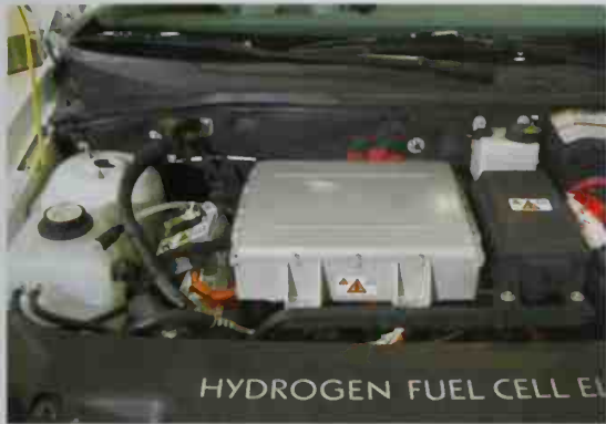
■ At a Volkswagen plant, a low-temperature fuel cell is given the final check prior to start-up, in order to ensure safety and efficiency.
