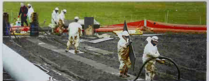
■ The cleaning up of oil spills along corroded pipelines is important to avoid soil contamination and the destruction of animal and plant habitats.
