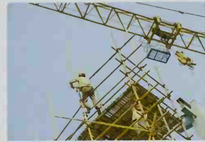
■ A Chinese construction worker goes about his work on a skyscraper under construction in the mega-city of Wuhan, central China's most populous city.
